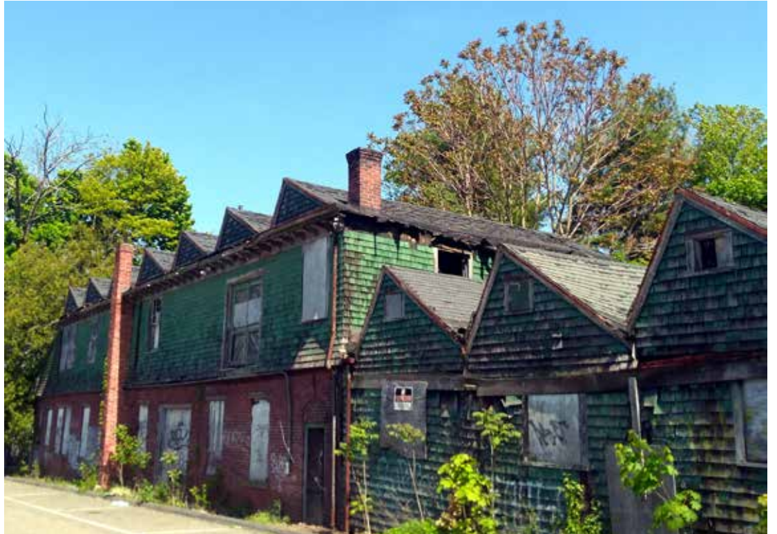
The Simon Laboratory. The building had what's called a "saw tooth" roof that had skylights to let fresh air and light into the rooms. Photo courtesy of Marilyn May.
