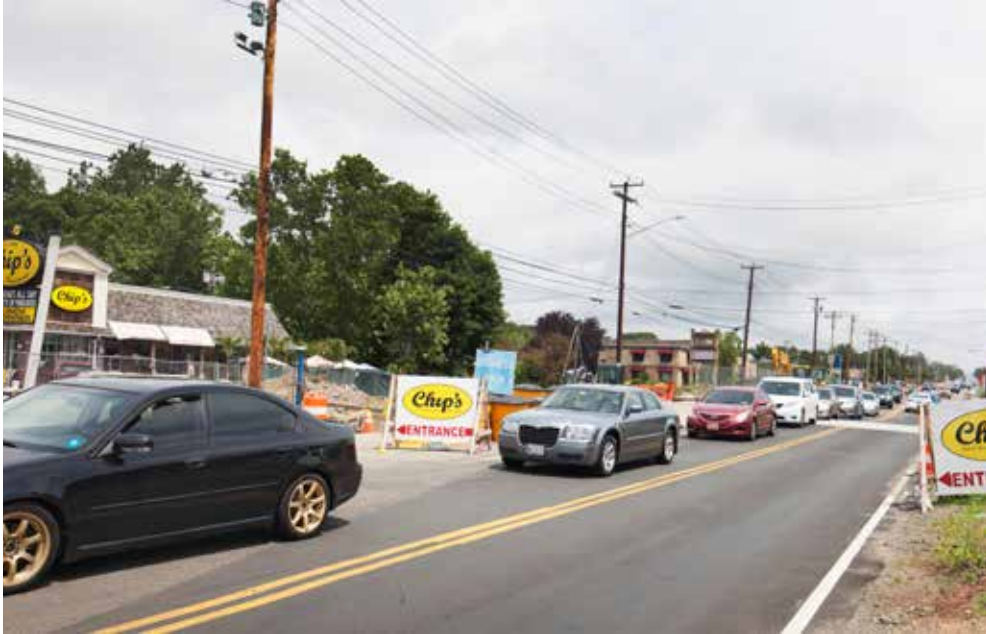
Cars line up along a stretch of the Boston Post Road in Orange where the road narrows to one lane in each direction for a construction project that will last until 2022. Photo by Steve Cooper.
