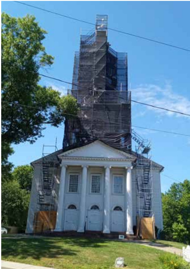
The steeple on the historic First United Church of Christ in Milford is undergoing renovations. Photo by Marilyn May.
